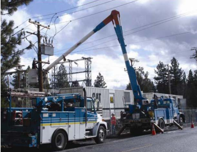
Figure 1: Cat XQ2000 Power Modules in Chester
