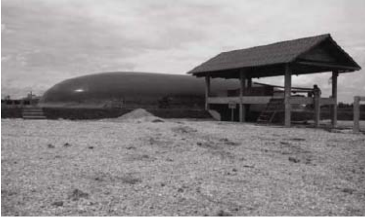
Figure 8: Buffer Tank and Digestion Process in Thailand
